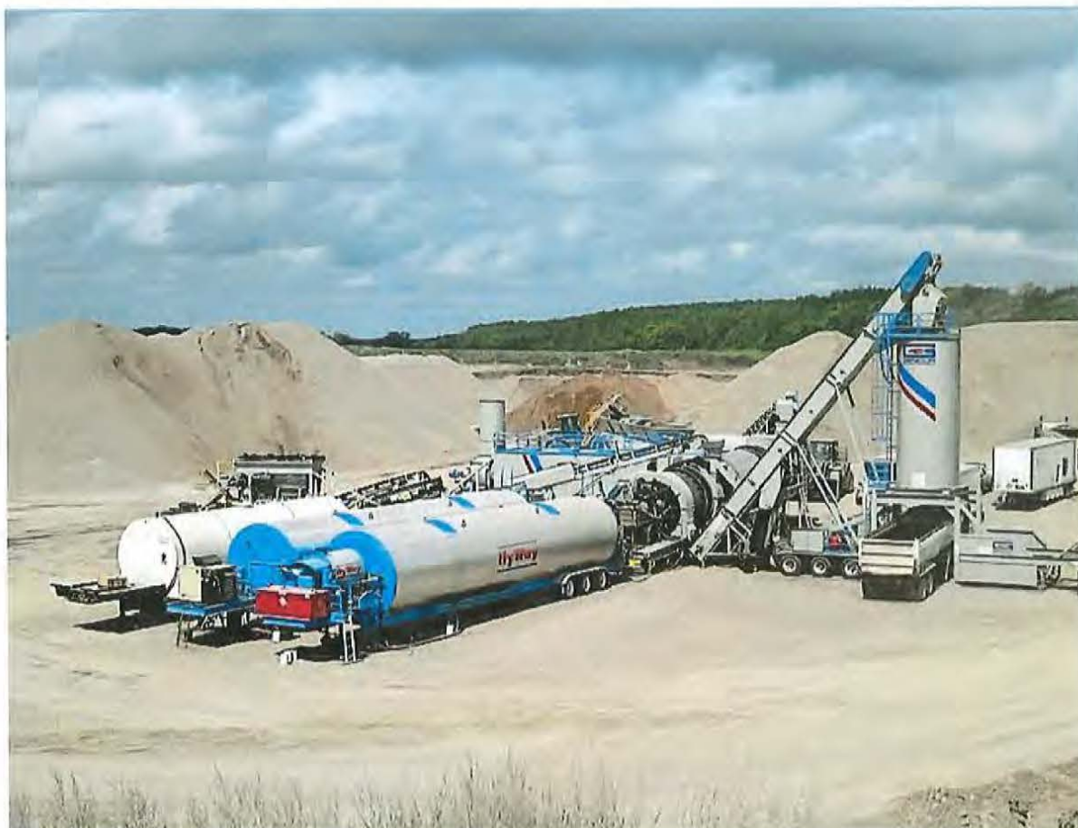
Figure 3 – Asphalt Drum Mix Plant (Typical) 1
