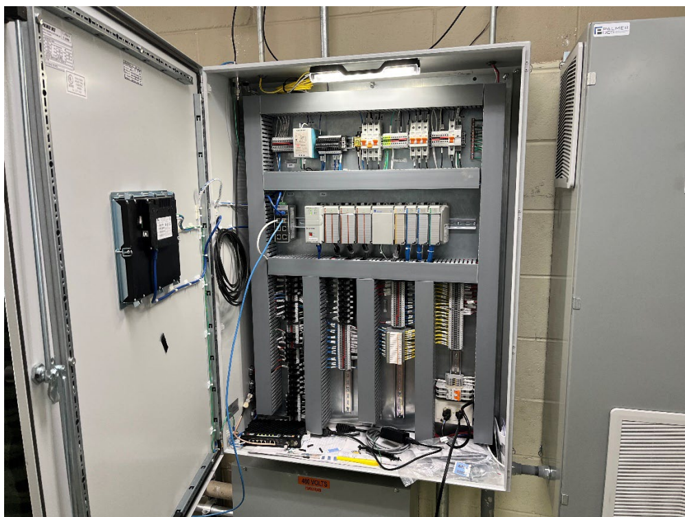
New PLC, about half the size and much cleaner!
