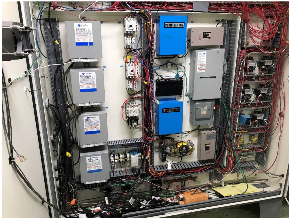
Old PLC Panel
