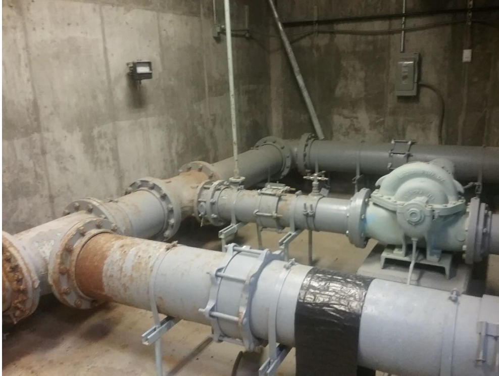
Old, unused process piping
